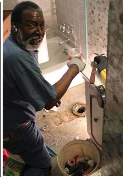
Local 189 member Bob Eskridge works on a house during the Christmas in April Charity event, now known as Rebuilding Together Central Ohio.
